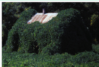
Kudzu Taking Over an Abandoned House in Mississippi, U.S.
